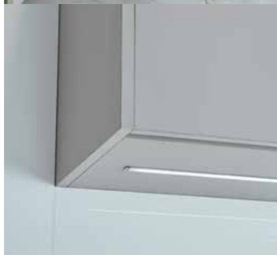
Recessed led lighting
